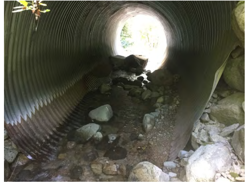
Material being washed into the culvert
